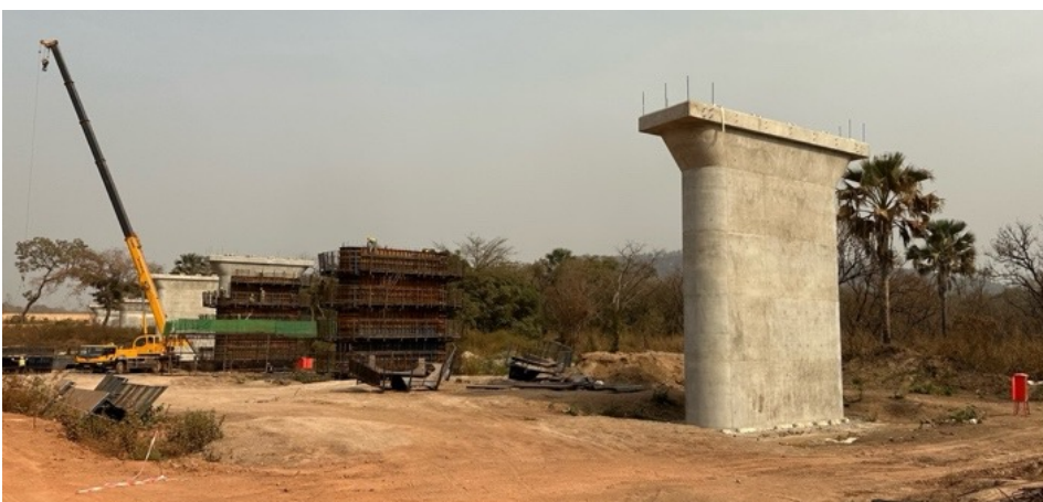
Measure 1.8: Construction of railway bridge in progress which also functions as a crossing for elephants.
