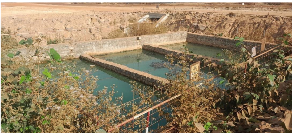
Measure 2.1: Effluent from a mixing station being pre- treated in a three-stage sedimentation tank before discharge.
