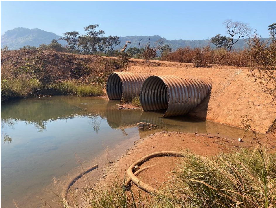
Measure 2.1: Stone masonry as a protective measure on slopes next to culverts.
