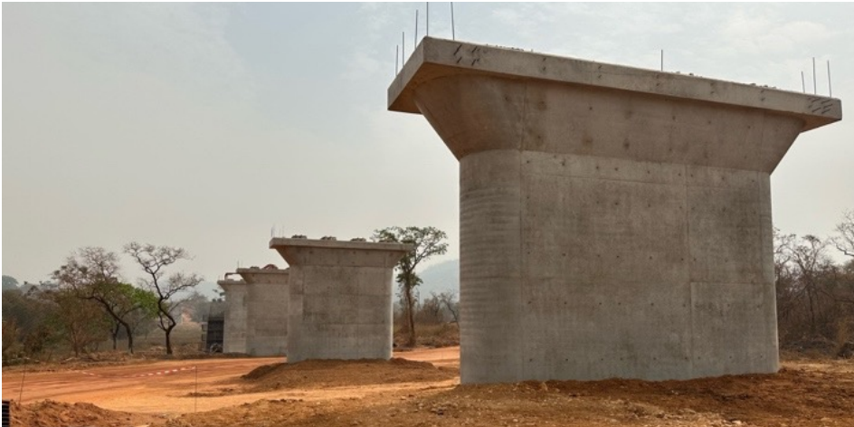
Measure 1.8: Construction of railway bridge in progress which also functions as a crossing for elephants.
