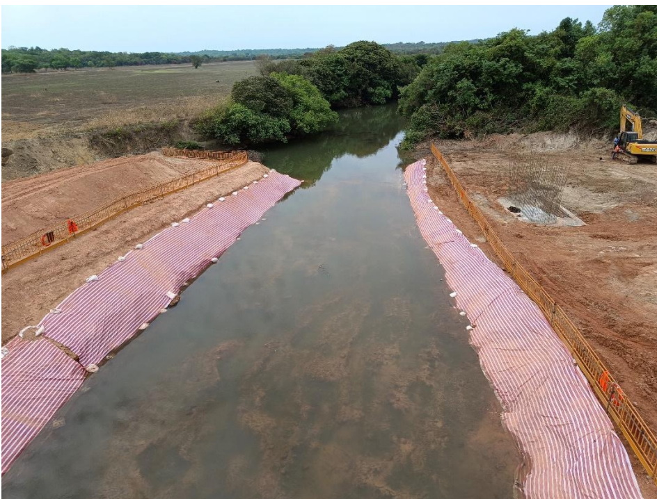
Measure 10.2: Anti-erosion protection measure on riverbank slopes of a bridge construction site.
